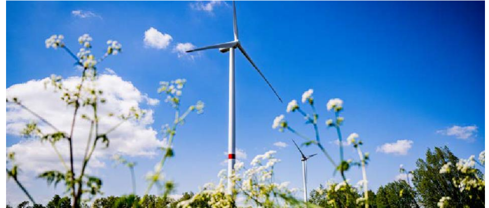
Storm Wind Belgium is a portfolio of onshore windfarms in Belgium. The portfolio consists of 56 turbines with a total capacity of approximately 185MW.
